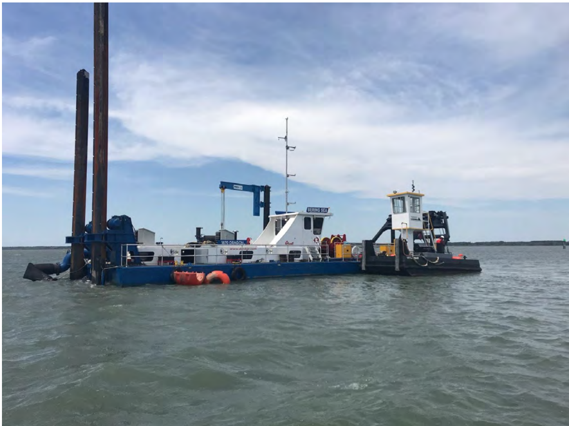
(Below) Photo 2: 2020 Hydraulic Dredge Plant, Bradford Bay, VA. Source Credits: USACE and SumCo Eco-Contracting
