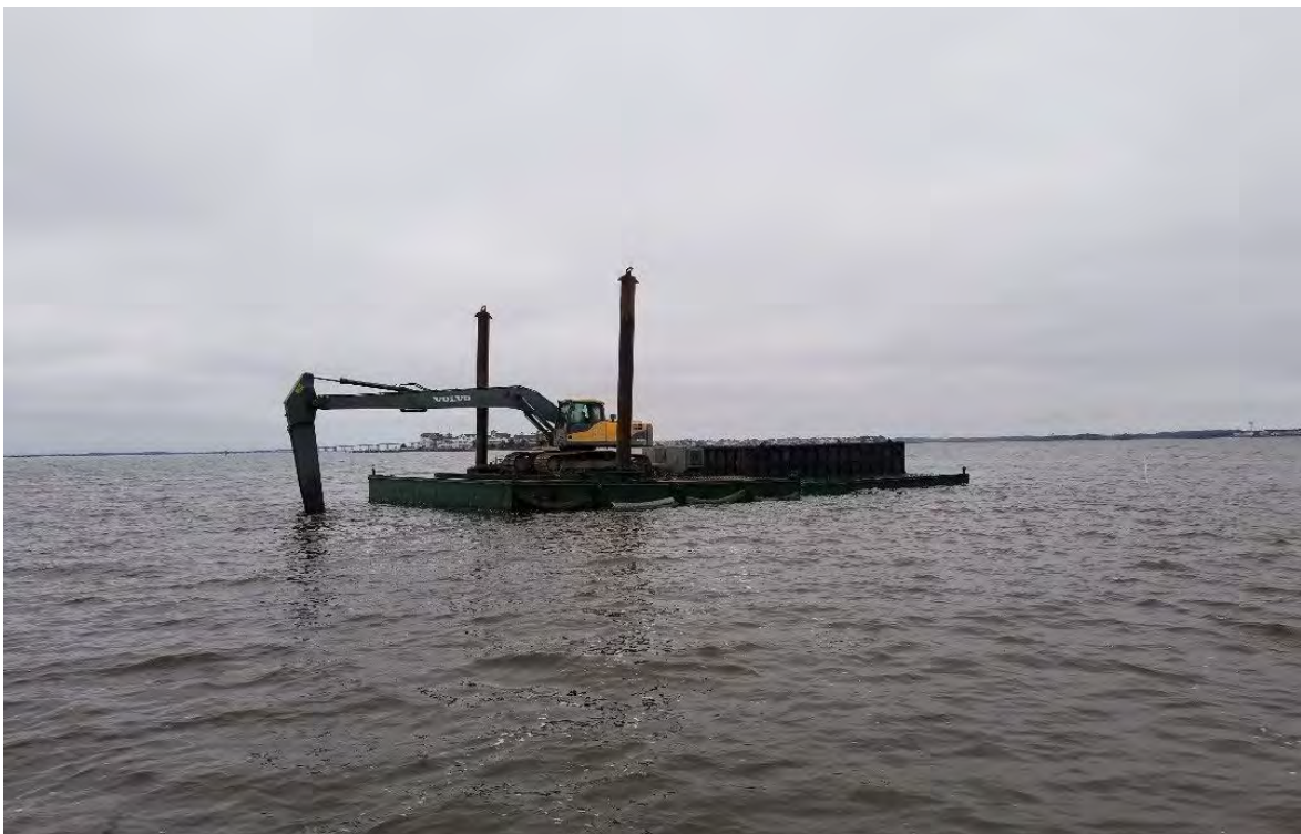
Photo 6: 2021 Mechanical Dredge Plant, Shallowbag Bay, NC. Source Credit: Dare County Grants and Waterways.
