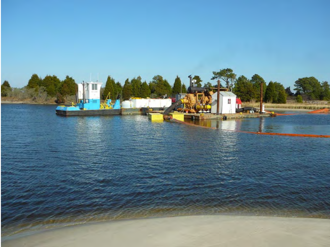
Photo 5: 2009 Hydraulic Dredge Plant, Winter Harbor, VA. Source Credits: USACE and Southwind Construction Corp.
